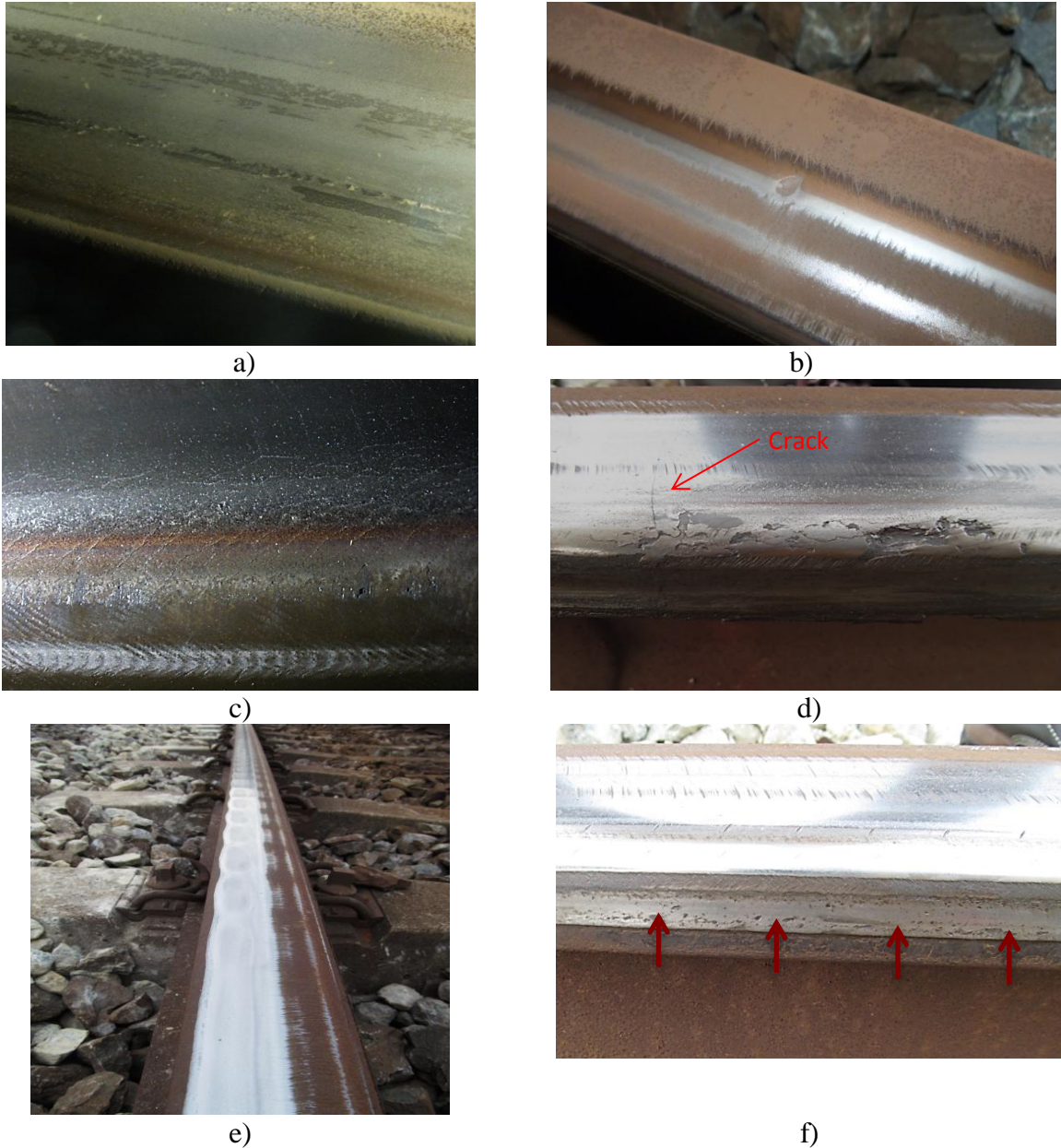
Figure 2. Common defects of the Metro of Medellín tracks. a) Adhesion, b) Class A – light Squat, c) Head checks, d) Spalling, e) Rolling contact Fatigue, f) Plastic flow.
