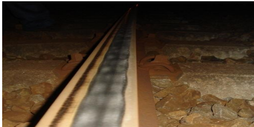
Figure 13. Rail corrugation in the Metro of Medellín.
