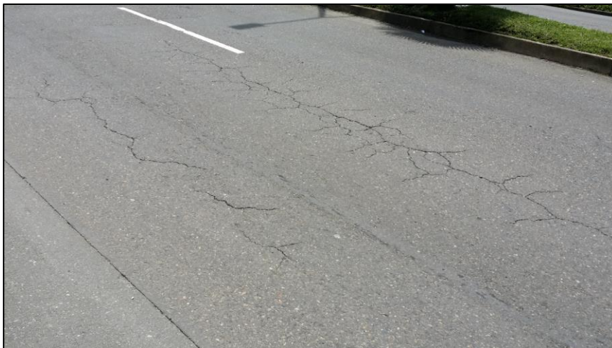
Figure 2-14: Cracking due to fatigue in asphalt pavements
