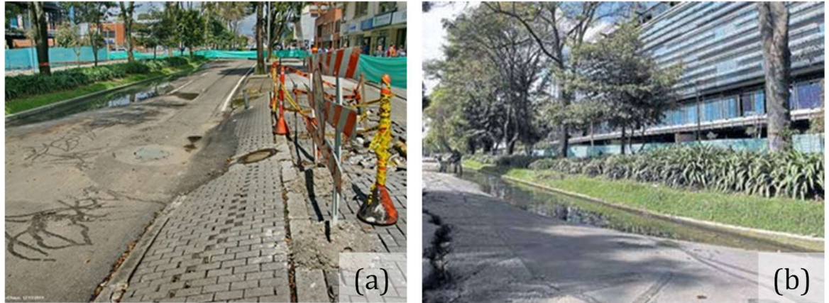
Photo 5-1. Settlement on 11th street. (a) impact on the vehicular roadway, and (b) impact on the pedestrian walkway. Photographs from Caracol Radio (2012) and Radio Santafe (2012).
