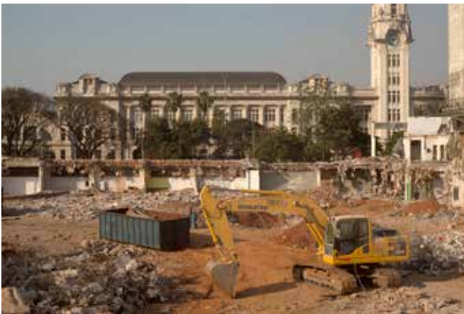
Image 5: Old bus station demolished. On site will be built the Dance Theatre. Photo: Eduardo Costa and André Kobashi 2011.
